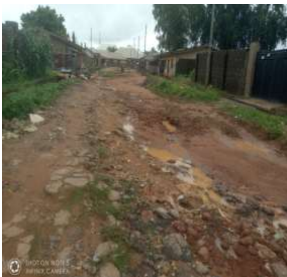
Plate 6: Status of Road during Rainy Season Sabo (Chikun LGA)
