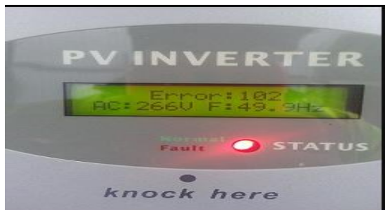
Figure 9: Solar Power Inverter (Agarwal et al. , 2017)
