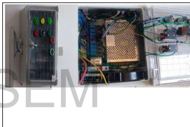
Fig. 2. Control unit with its components.
